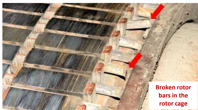
Fig.1 Example of rotor fault in a 320 kW motor operating in a mining facility.
