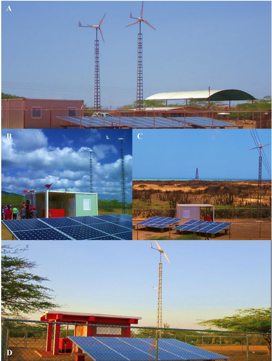
Figure 6. Examples of hybrid microgrids of different architectures: (A) SH-40 in Cusia, (B) SH-30 in Wososo, (C) SH-20 in La Macolla and (D) SH-10 in Jacuque
