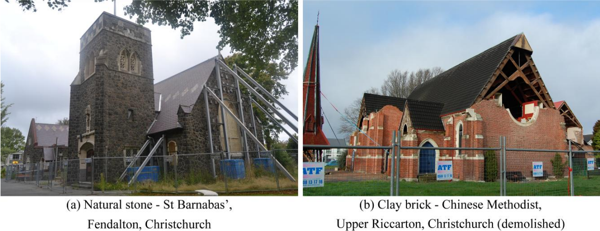
Figure 3.2. Examples of building materials of the URM churches in the Canterbury region. Photo (b) is courtesy of João Leite.
