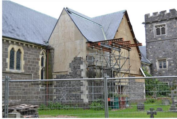
(b) Overturning of the transept - St. Peter's, Upper Riccarton, Christchurch
