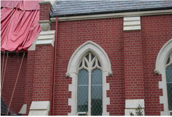
(a) Shear in the longitudinal walls - Our Lady Star of the Sea, Sumner, Christchurch
