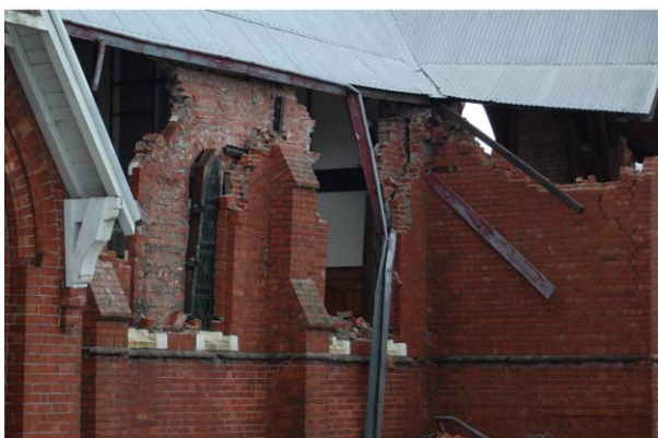
(c) Church of the Good Shepherd, Phillipstown, Christchurch (demolished)
