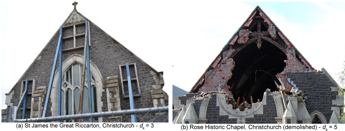
Figure 3.4. Examples of damage ascription for mechanism no. 2 (gable mechanisms). Photo (b) is courtesy of João Leite.
