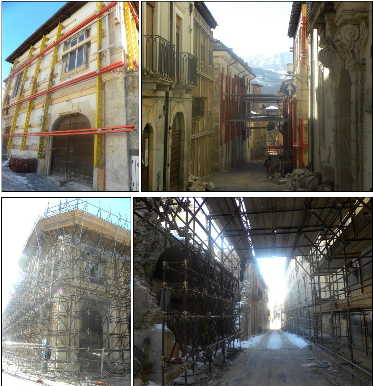
Figure 2. Complex expensive propping works of single structures (photos on the left) and among facing buildings (photos on the right) in L'Aquila. Photos: C. Pesaresi (February 2010).
