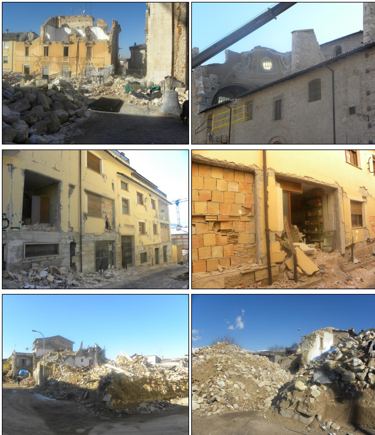
Figure 1. Huge damage to buildings and church roofs and the top of the walls (photos above) in L'Aquila; damage above all to the medium-low floors and failure of the external lining (photos in the center) in L'Aquila (and overturning of parts of walls in the photo on the left – at bottom); notable phenomena of collapse at Onna (photos below), a hamlet of L'Aquila. Photos: C. Pesaresi (February 2010).
