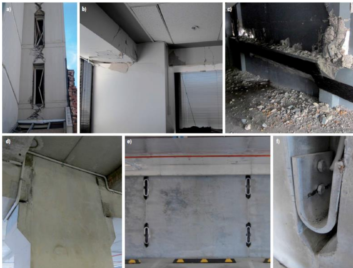
Figure 15: Ductile-response RC systems: a) coupling beams of 1960s coupled-walls building; b) beam plastic hinges on 1980s perimeter RC frames building; c) ductile behaviour of 1980s RC walls building and d–f) “low-damage” PRESSS post-tensioned frames building built in 2010 (photos from Kam and Pampanin [29]).
