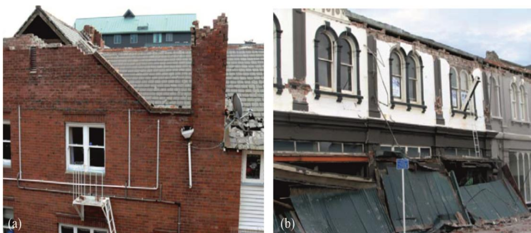
Figure 9: (a) Examples of chimneys and gable wall and (b) parapet failure observed in clay brick URM buildings during the Sept. 4, 2010 Darfield earthquake (photos from Ingham and Griffith [26]).
