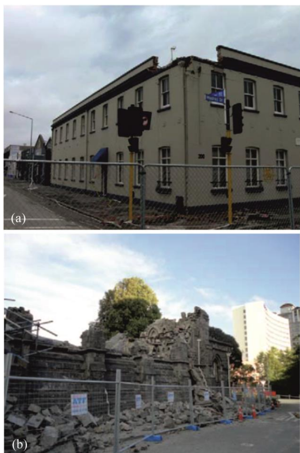
Figure 12: (a) External view of failed parapet at corner; (b) collapse of the Stone Chamber of the Canterbury Provisional Chambers building. Photos from Ingham and Griffith [26].
