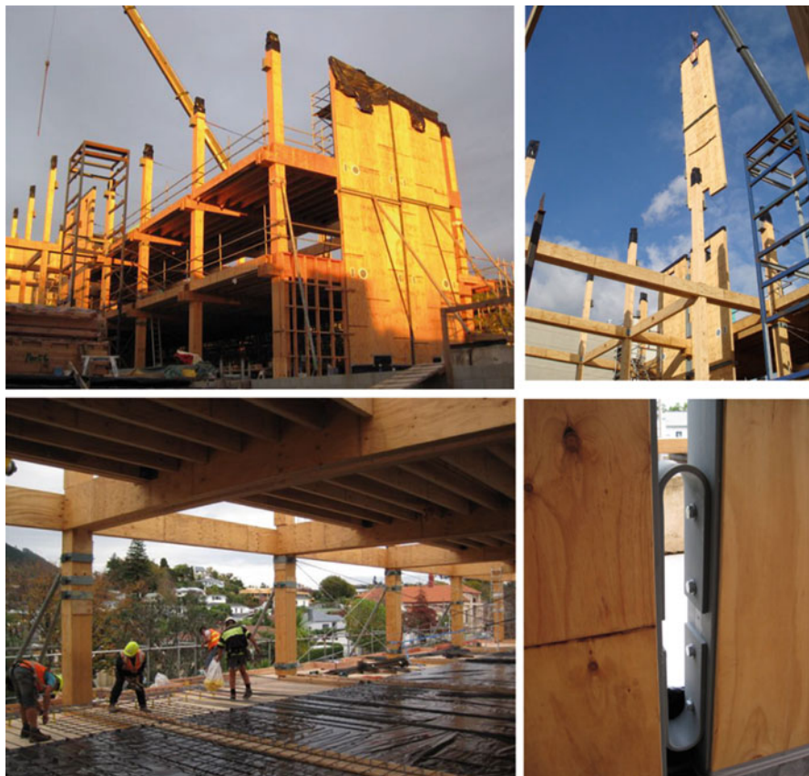
Fig. 13.27 Nelson Marlborough Institute of Technology, (NMIT), Nelson, New Zealand. Post-tensioned timber (Pres-Lam) walls coupled with UFPs (Structural Engineers Aurecon; Architects Irving-Smith-Jack, Devereux et al. 2011)
