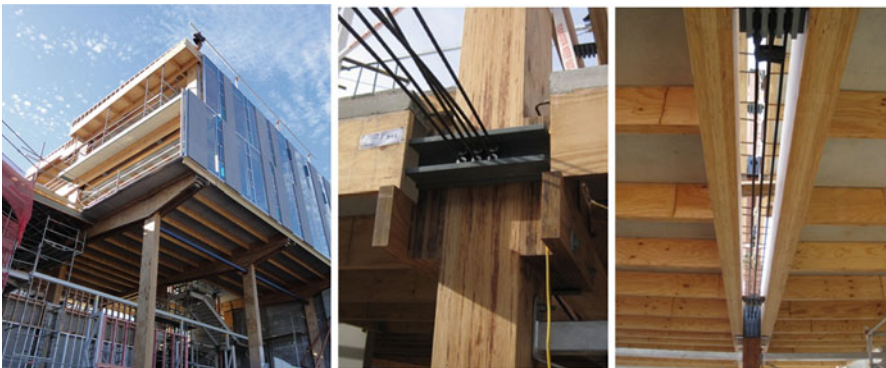
Fig. 13.30 College of Creating Arts – MacDiarmid Building, Massey University, Wellington, New Zealand. Post-tensioned timber (Pres-Lam) frames in the transverse directions with horizontal U-Shape flexural plate dissipaters on the first floor and Post-tensioned concrete (PRESS) walls in the longitudinal direction (Structural Engineers: Dunning Thornton Consultants)
