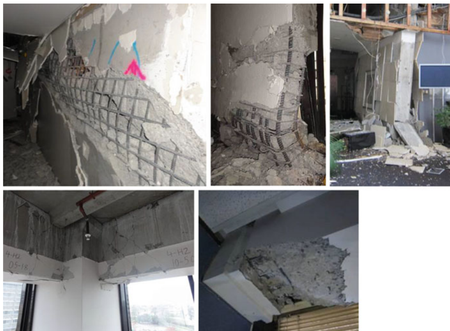
Fig. 13.3 Example of damage to RC frames and walls (all these buildings have been demolished) (From Kam et al. 2011; Pampanin 2012)
