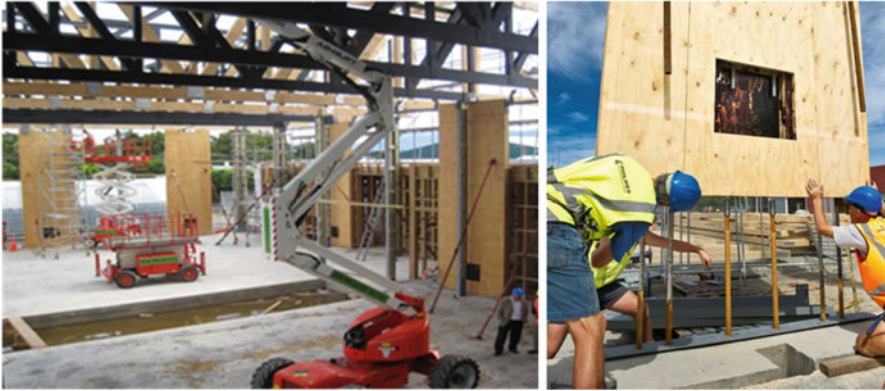
Fig. 13.28 Carterton Events Centre, New Zealand. Single-storey building with LVL truss roof (Designed by Opus International: Dekker et al. 2012)
