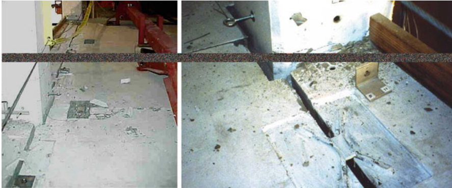
Fig. 13.15 “X-connectors” between precast floor (pre-topped double-tee) units and frames as implemented in the PRESS Five Storey Building (Priestley et al. 1999)
