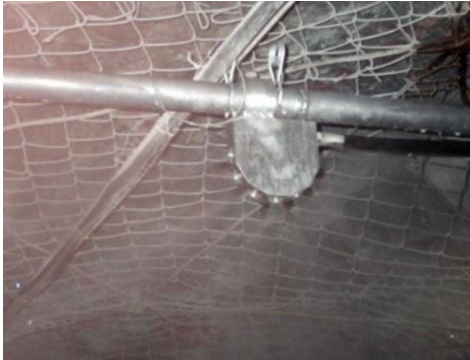
Figure 3: Spray heads utilised for the spray system.
