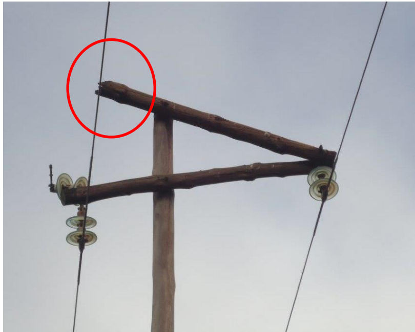
Figure 1.2: Typical example of a burnt structure in the field [4]
