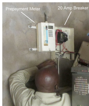
Fig. 1. A typical installation showing the pre-payment meter and 20A breaker.
