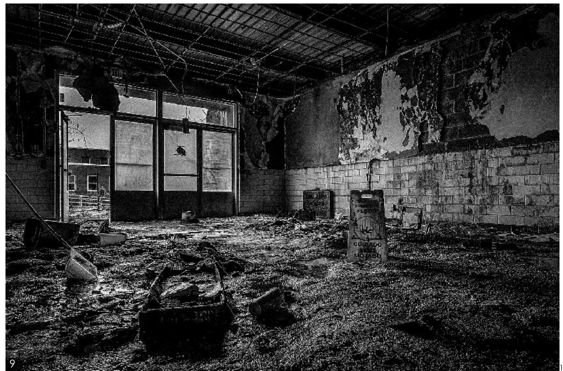
Figure 8, 9: Images of sites which were old asylums and rehabilitation facilities now neglected and run down.
