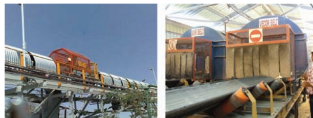
Figure 3—Go-belt sampler installation on conveyor belts from shaft head (source: Letsie, 2009; Minnitt, 2013)
