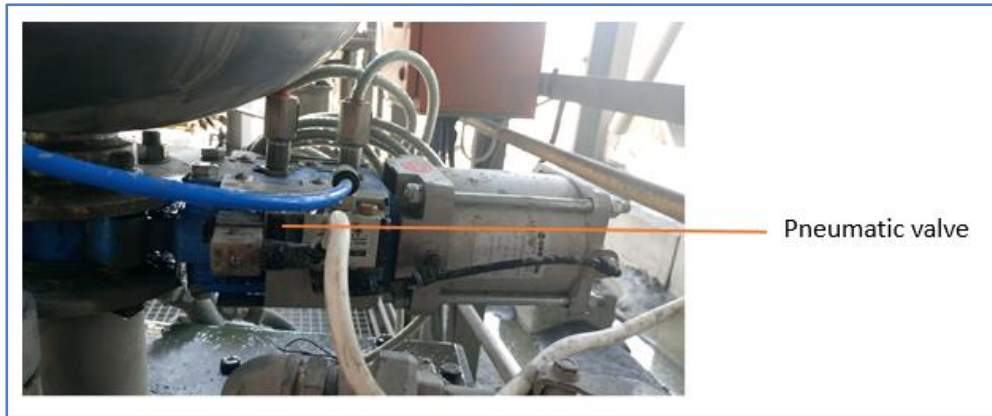
Figure A.17: Pneumatic Valve at Hopper Discharge End.
