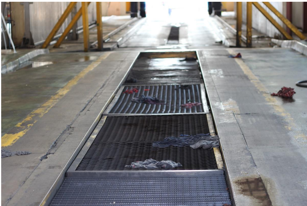
Appendix ii: Spills on site are not well managed, and are soaked up fibre cloths
