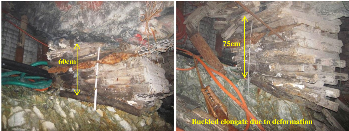
Figure 37. Minimal deformation observed on the packs in the W6 cleaning gully.
