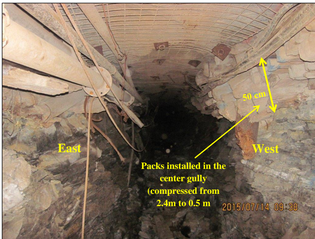
Figure 60. Photo of the 104-66 Raise. The pack on the raise shoulders were installed with a full cut ledge at 2.4m high and currently measure only 0.5m in height.
