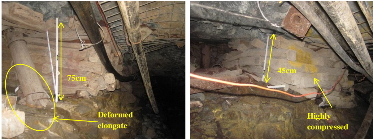
Figure 32. Photos of the E8 gully cleaning gully showing deformed support
