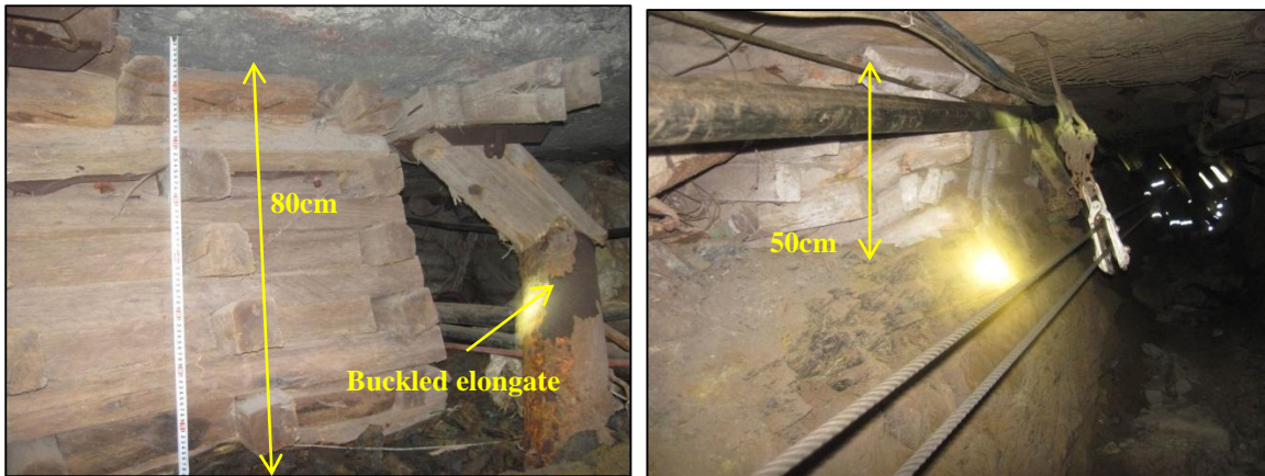
Figure 29. Closure observed on timber pack and elongates in the W11 cleaning gully.
