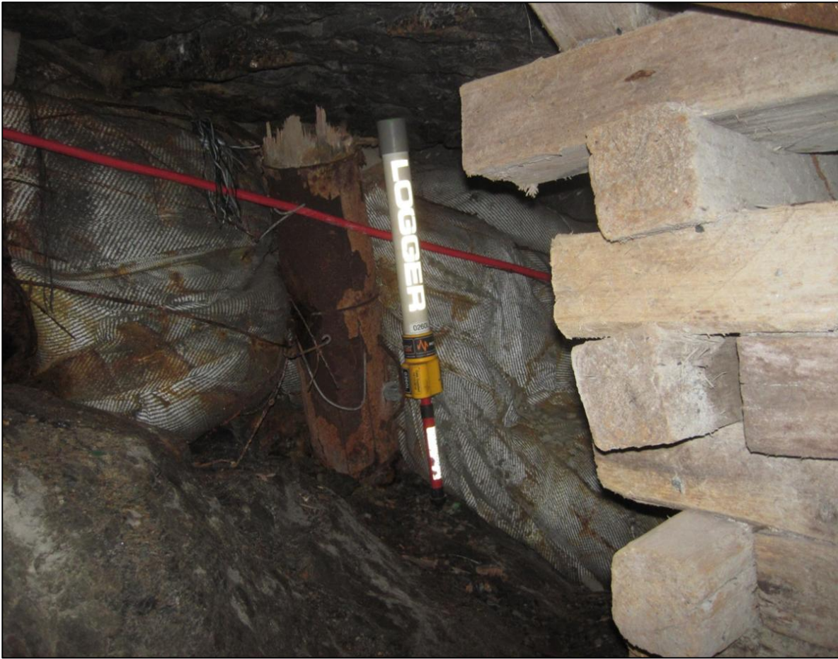
Figure 25. Logger 260 installed on the North shoulder of the W9 cleaning gully
