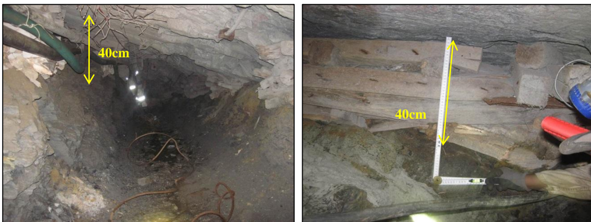
Figure 30. Closed gully shoulders and highly deformed timber packs in the W10 gully.
