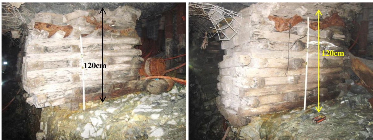
Figure 38. Little signs of deformation on the timber packs in the W7 cleaning gully.
