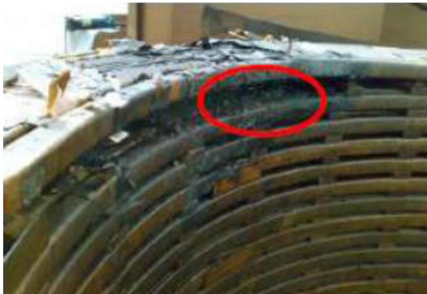
Figure 1.3: TresMarias Substation: Failed 25 MVA, 13.8/289 kV step-up transformer (courtesy of Angelica da Costa Oliveira Rocha)
