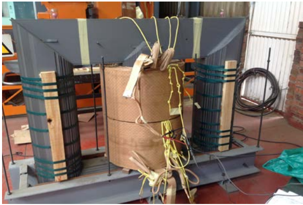
Figure 10a: Split MV winding transformer
