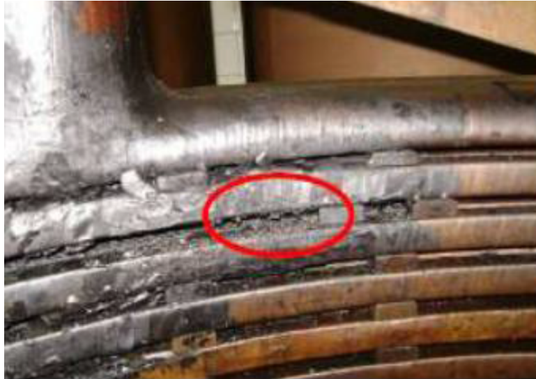
Figure 1.2: TresMarias Substation: Failed 25 MVA, 13.8/289 kV step-up transformer (courtesy of Angelica da Costa Oliveira Rocha)
