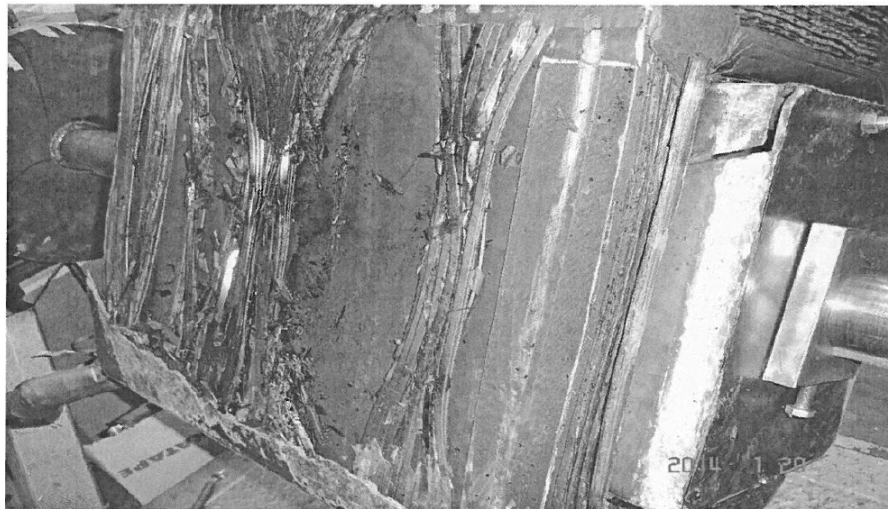
Figure 1.4: Failed winding with inter-turn insulation severely damaged (courtesy of Transformer Manufacturer)
