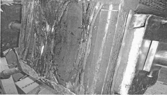
Fig. 1. Failed winding with inter-turn insulation severely damaged.
