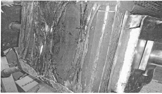
Fig. 1. Failed winding with inter-turn insulation severely damaged
