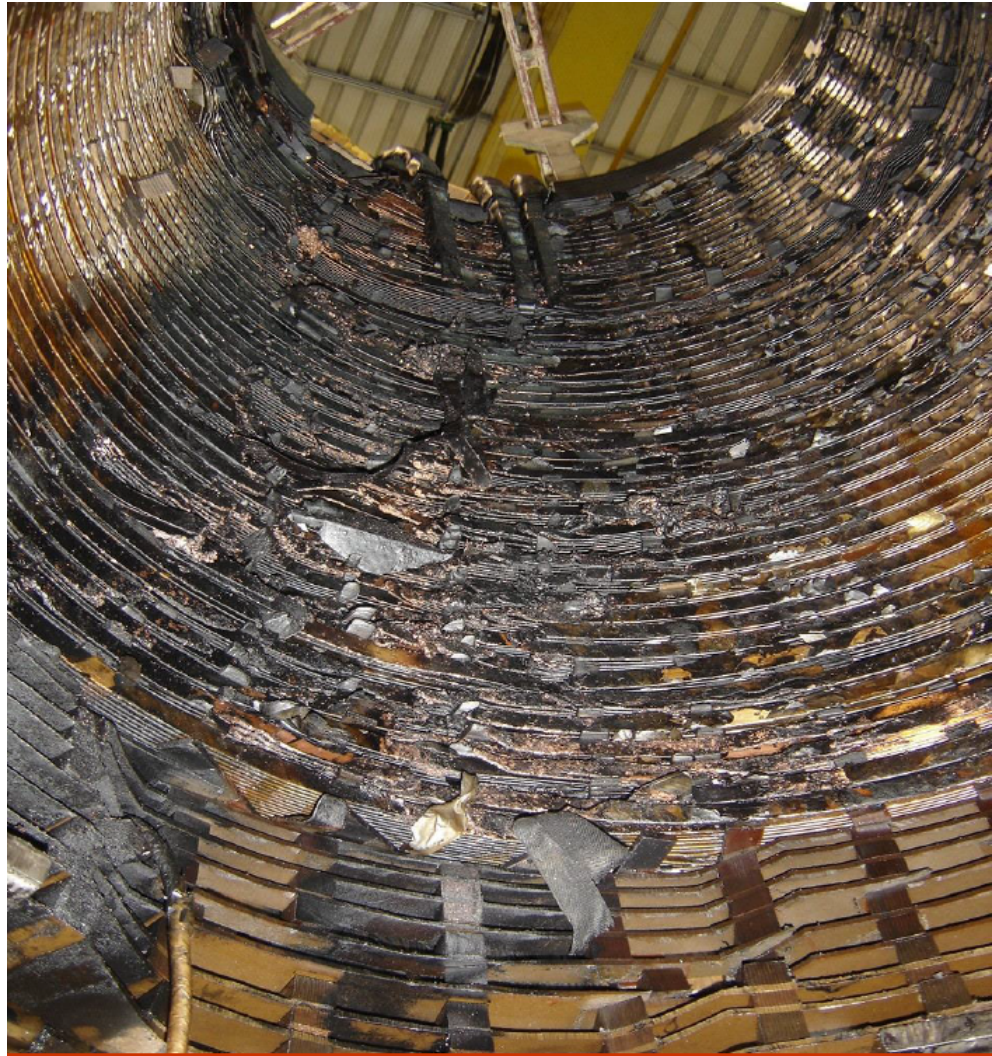
Figure 1.1: Failed SE Ipatinga 1 Autotransformer 230/161/13.8 kV (courtesy of Angelica da Costa Oliveira Rocha)
