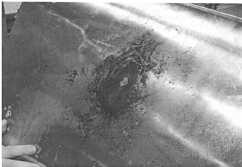
Figure 1.6: Burning of first layer of LV foil winding (courtesy of Transformer Manufacturer)
