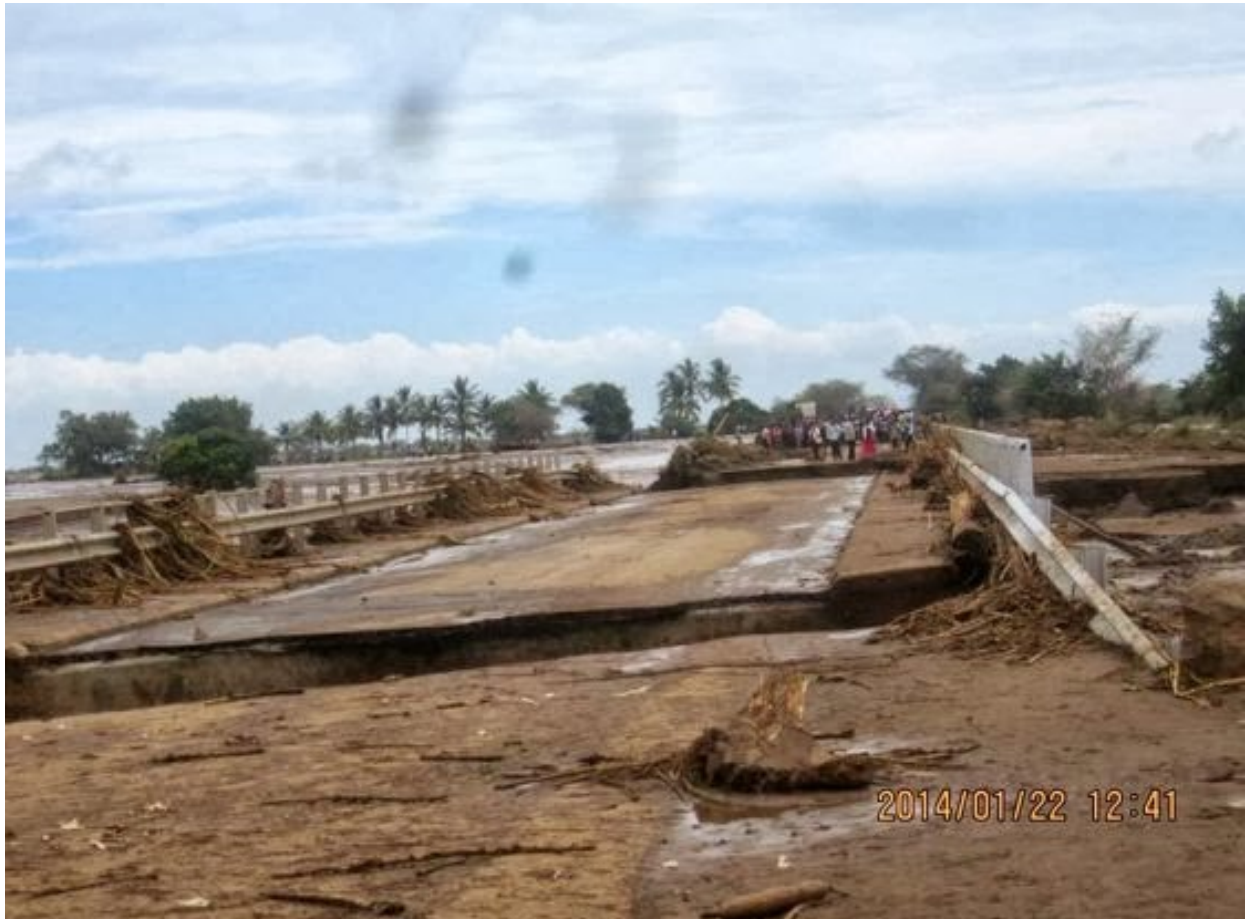
Figure 5.2: The Dumila area bridge after heavy rainfall, on 22-01-2014. Source: Michuzi Blog - http://issamichuzi.blogspot.com/
