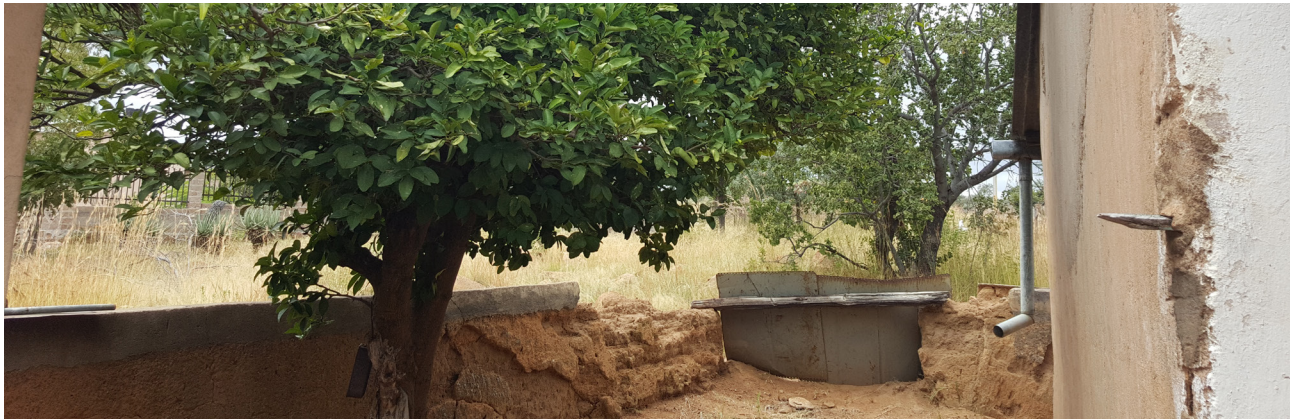
The damaged old daga at the back of the lapa .
