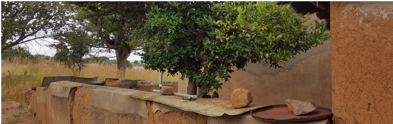
The old daga walls were plastered in cement plaster to try protect them from rain, now metal sheeting has been loosely placed for the same reason.
