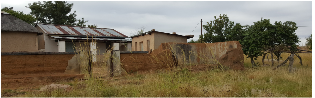
The combination of thatched and corrugated roof sheeting was used, projecting the building of the different huts at different times.
