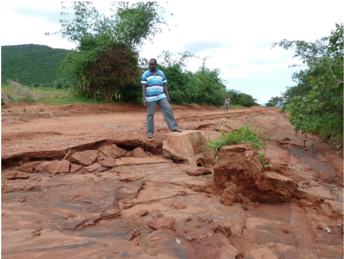
Plate 5.3: Section of the road destroyed by excessive rain at Ikuvala village
