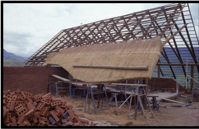
Figure 4.3: The early stages of construction of the Kamberg Rock Art Centre and the complete building.
