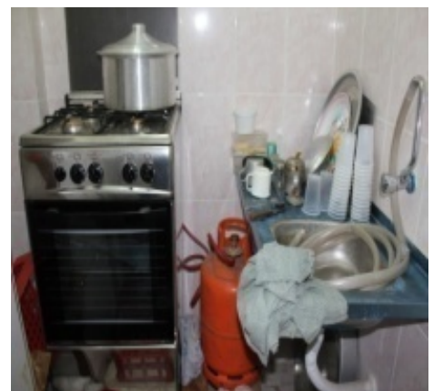
Figure 6.41 Kitchen with cooker and sink gas supply just visible in this crowded space
