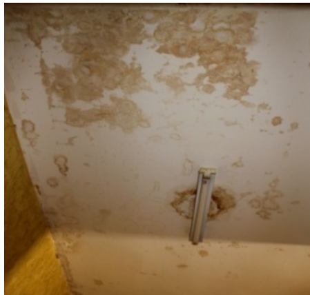
Figure 6.63 Shows water damage and peeling paint on the ceiling
