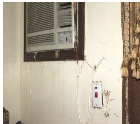
Figure 6.64 Photos show ceiling in the bathroom and kitchen is peeling and damaged, also exposed wires from the air conditioning unit where dripping water can build up
