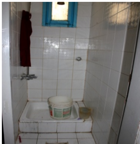
Figure 6.52 Shows bathrooms on the ground floor, there are cockroaches on the floor
