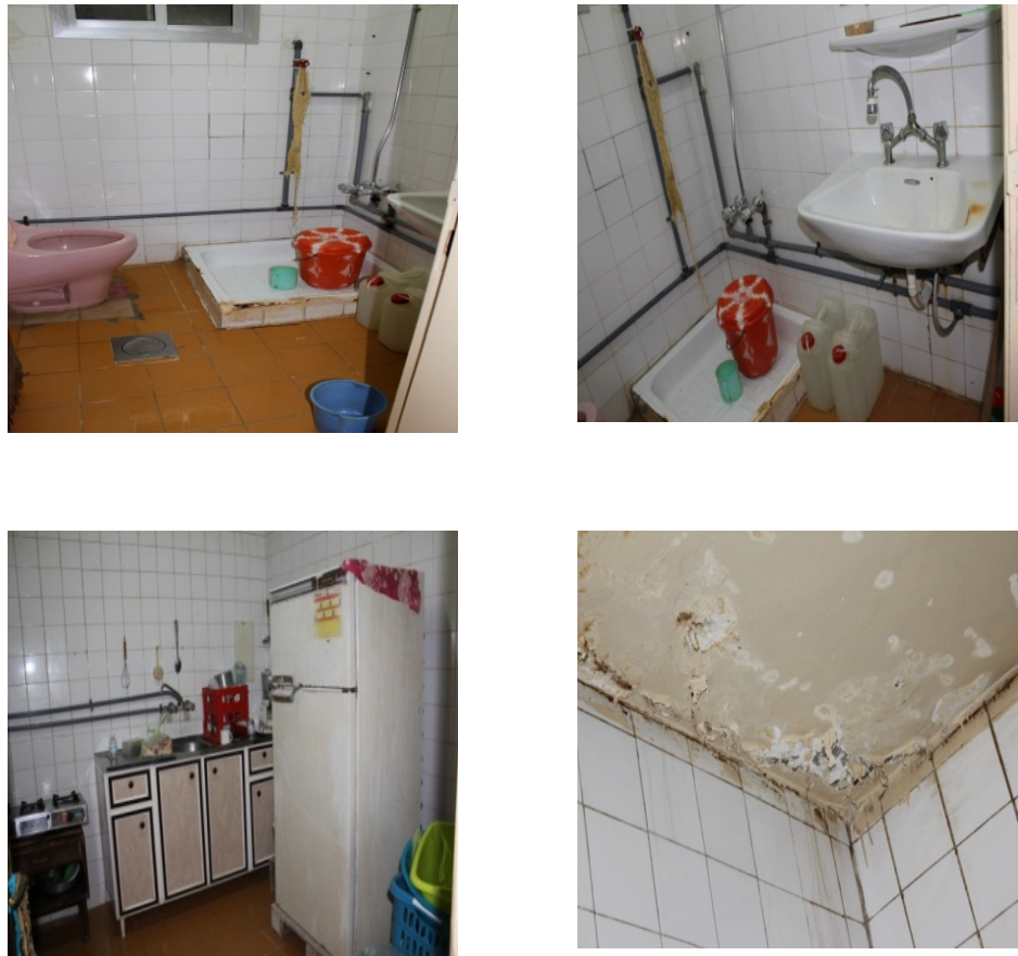
Figure 6.81 Photos show the dire condition of a bathroom and a kitchen, here too, the bathroom is not fitted for the needs of disabled residents
