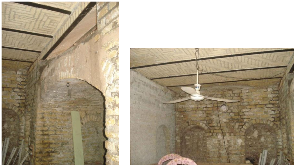
Figure 7.4: High humidity affecting the walls of the sardab in the T.C.H.T in the Al-Kadhimiya, House NO.4 (PH. CH4, 2012), (Author).
