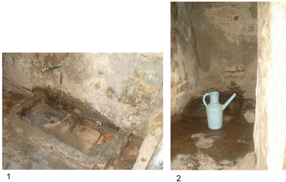
Figure 7.27: The high humidity affects the ground floor, House NO. 12 (PH. CH12, 2012), (Author). (1) Courtyard (2) The service spaces
