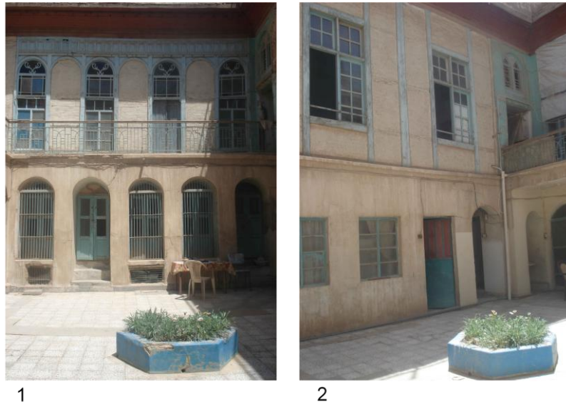
Figure 7.7: Refurbishing the T.C.H.T in Al-Kadhimiya, House NO.2 (PH. CH2, 2012), (Author) by: (1) Courtyard floor covered by ceramics, with the fountain now a flowerbed; (2) Establishing new drainage pipes and new electrical wiring
