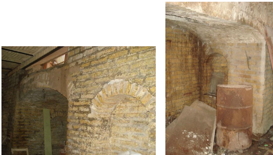
Figure 8.4: The abandoned sardab as a result of the high humidity and odours in the T.C.H.T in the Al-Kadhimiya (PH, CH7, 2012), (Author).
