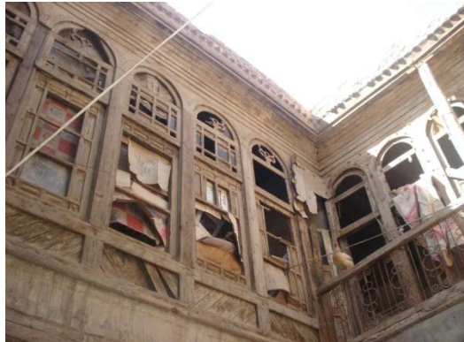
Figure8.15: The lack of maintenance of the T.C.H.T in the Al-Kadhimiya led to an uncomfortable environment (PH, CH 12, 2012), (Author)
