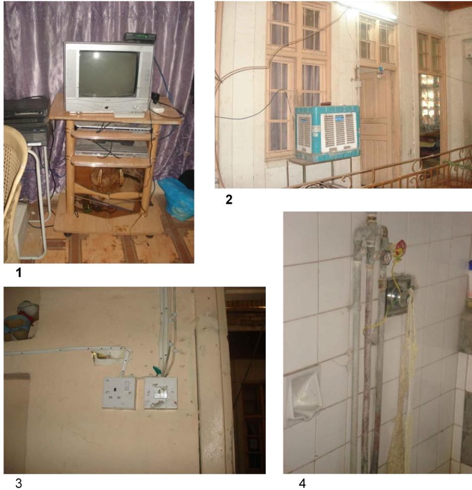
Figure 7.14: Example of refurbishing and types of device in the T.C.H.T in Al-Kadhimiya, House NO. 6 (PH. CH6, 2012), (Author):
