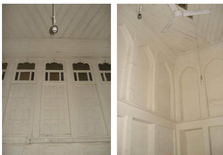
Figure 8.9: Types of refurbishment of the T.C.H.T by painting the walls every two years (PH, CH.8, 2012), (Author)
