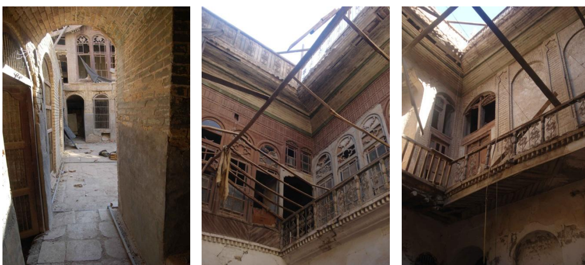
Figure 8.24: Damage to the large part of the house with the big courtyard in the Al-Kadhimiya (PH, CH9, 2012), (Author).
