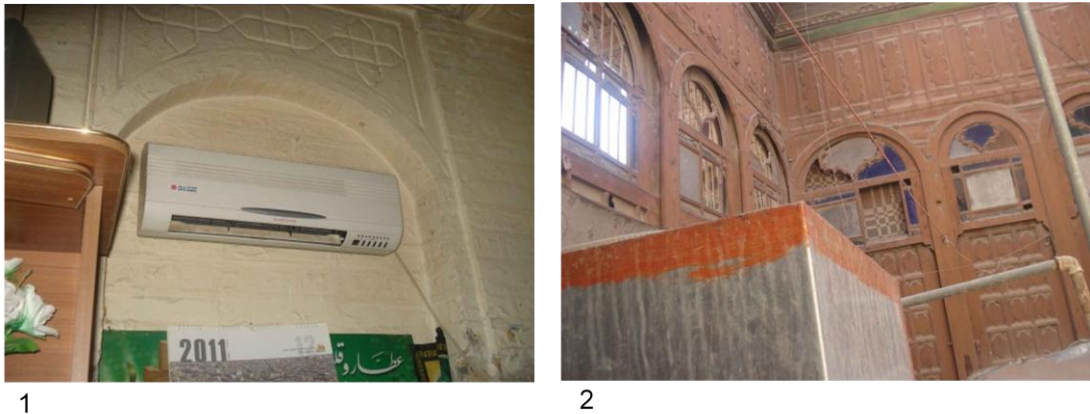
Figure 7.21: Example of different devices in the T.C.H.T in Al-Kadhimiya, House NO. 9 (PH. CH9, 2012), (Author (1) Adding a split unit on the ground. (2) Adding a water tank on the first floor
