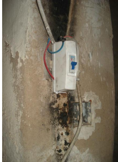
Figure 9.15: Safety issue show the potential fire hazard during the changes in the electricity supply current as an environmental challenge in the T.C.H.T. in the Al-Kadhimiya (PH.CH.6, 2012), (Author).
