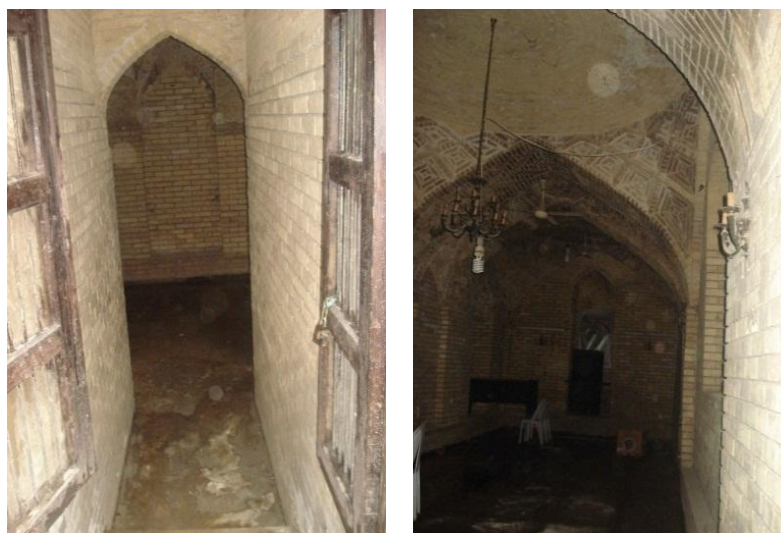
Figure 6.5: The weakness such as difficulty to control of underground water in sardab of T.C.H.T that arise according to the modernization (PH, CH10, 2012), (Author).
