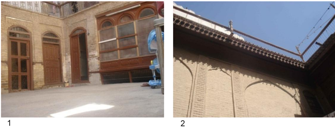
Figure 7.2: Refurbishing a T.C.H.T in Al-Kadhimiya, House NO.1 (PH. CH1, 2012), (Author) by: (1) Courtyard floor covered by cement, with painted windows and doors; (2) Covered walls, and establishing a new drainage pipe.
