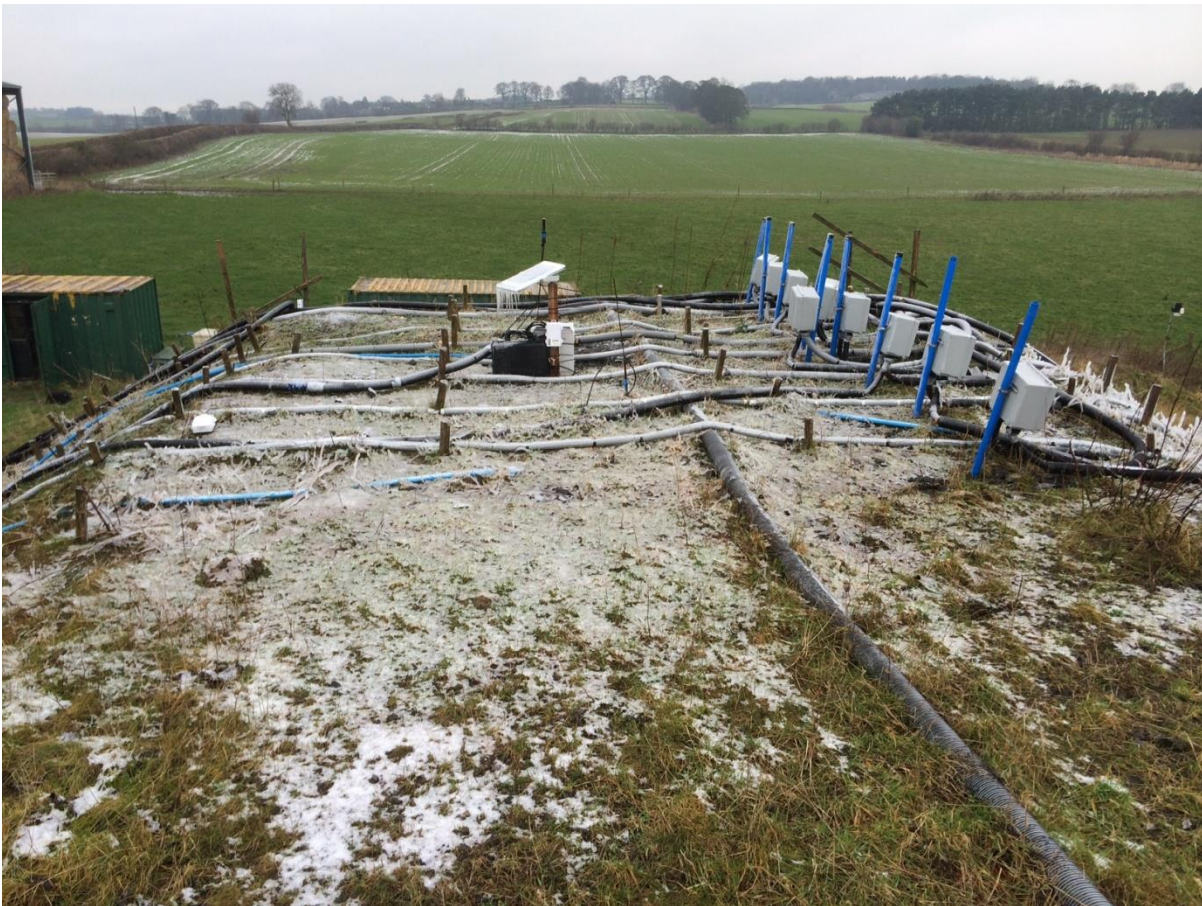
Figure 5.61 Frozen sprinkler water at on the embankment surface
