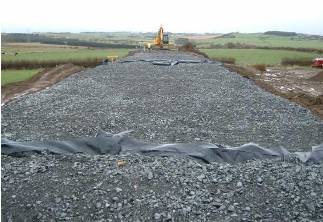
Figure 3.11 Granular capping layer on the BIONICS embankment crest . The hydrologically-isolating Visqueen layers can be observed
