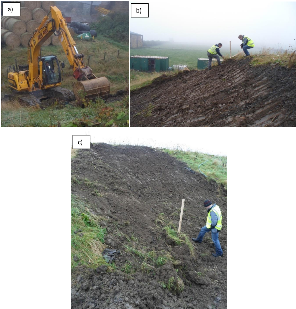
Figure 4.34 Slope steepening of the ERT test plot section of the BIONICS embankment, showing (a) regrading using a JCB; (b) angle measuring of regraded slope; (c) after the replacement of topsoil to encourage vegetation growth
