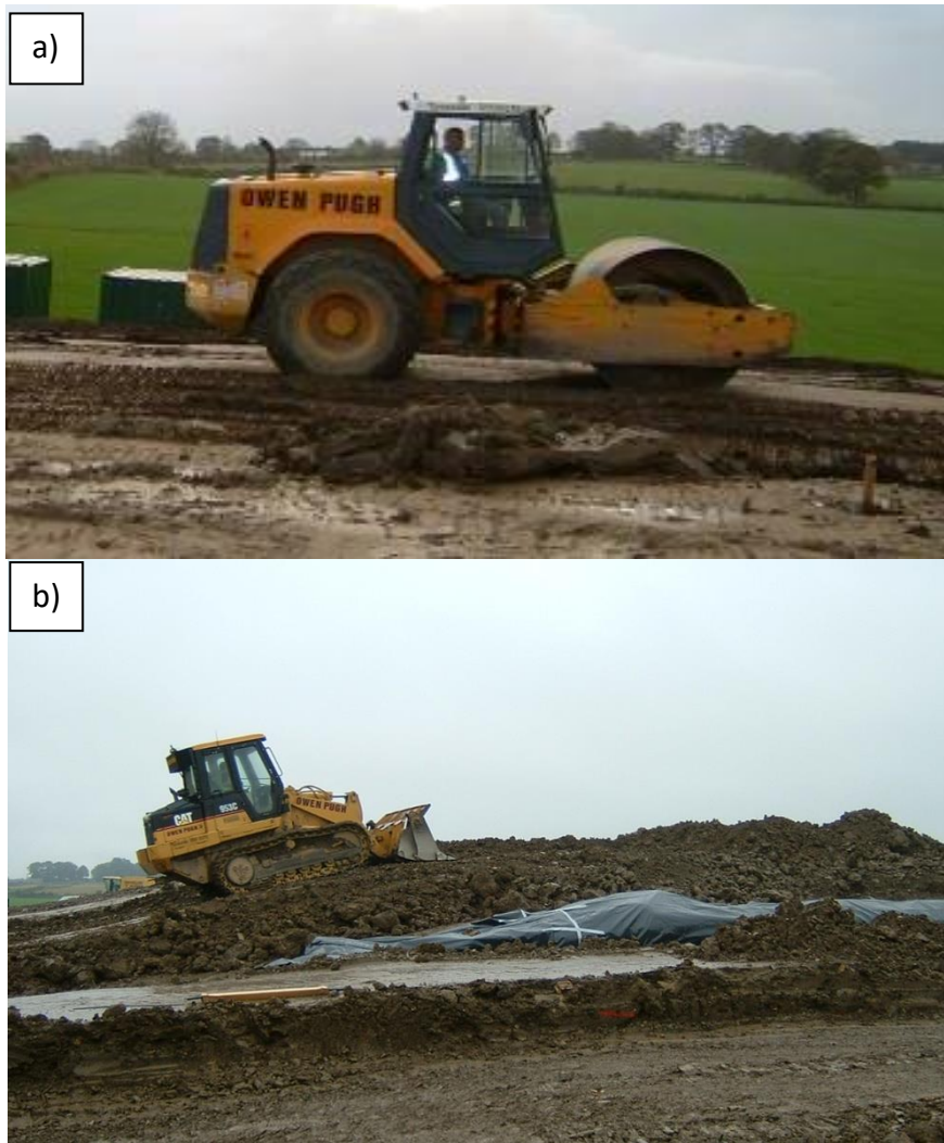
Figure 3.8 Embankment compaction methods (a) self-propelled roller used on well-compacted panels; (b) plant used on poorly-compacted panels (image taken from Hughes et al., 2009)
