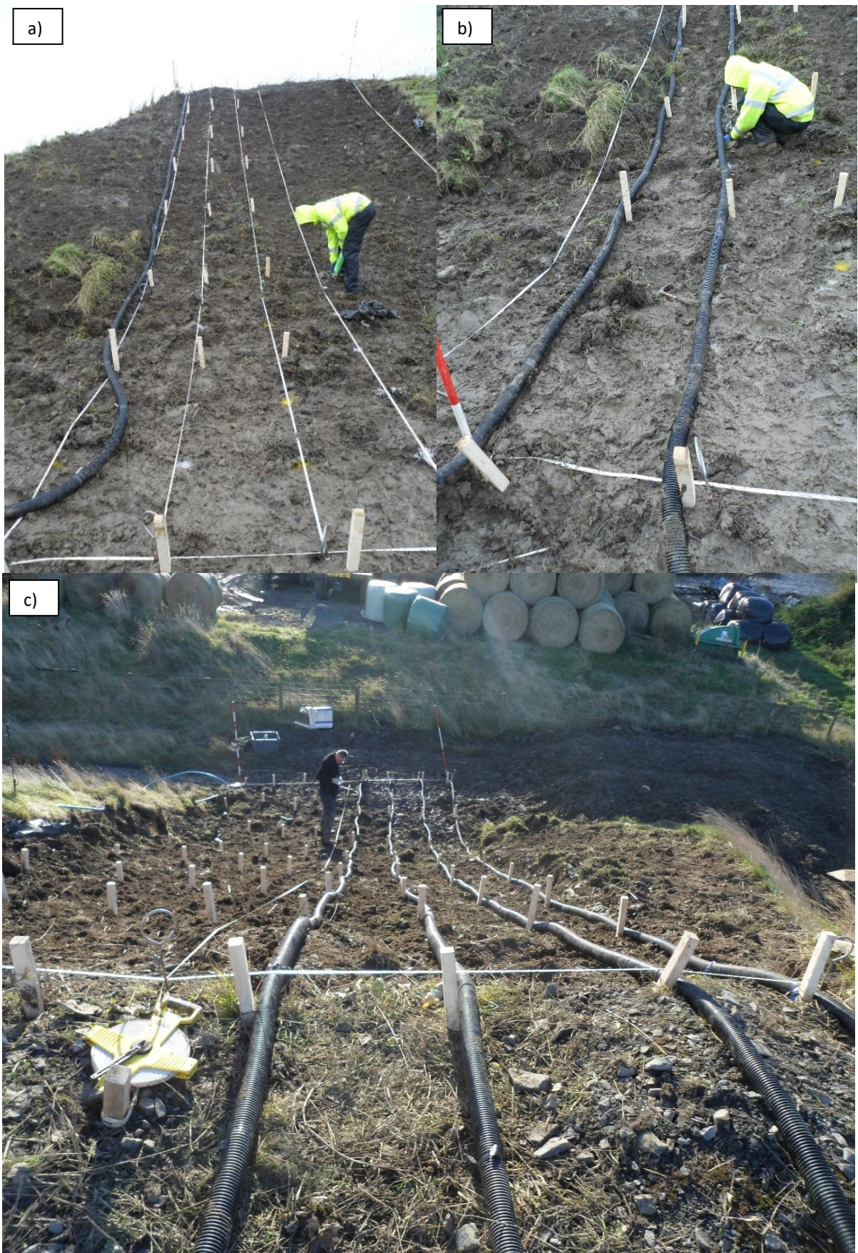
Figure 4.42 Installation of 3D ERT array. (a) wooden stakes and measuring tapes for marking electrode positions; (b) installation of electrodes; (c) view of installation from crest
