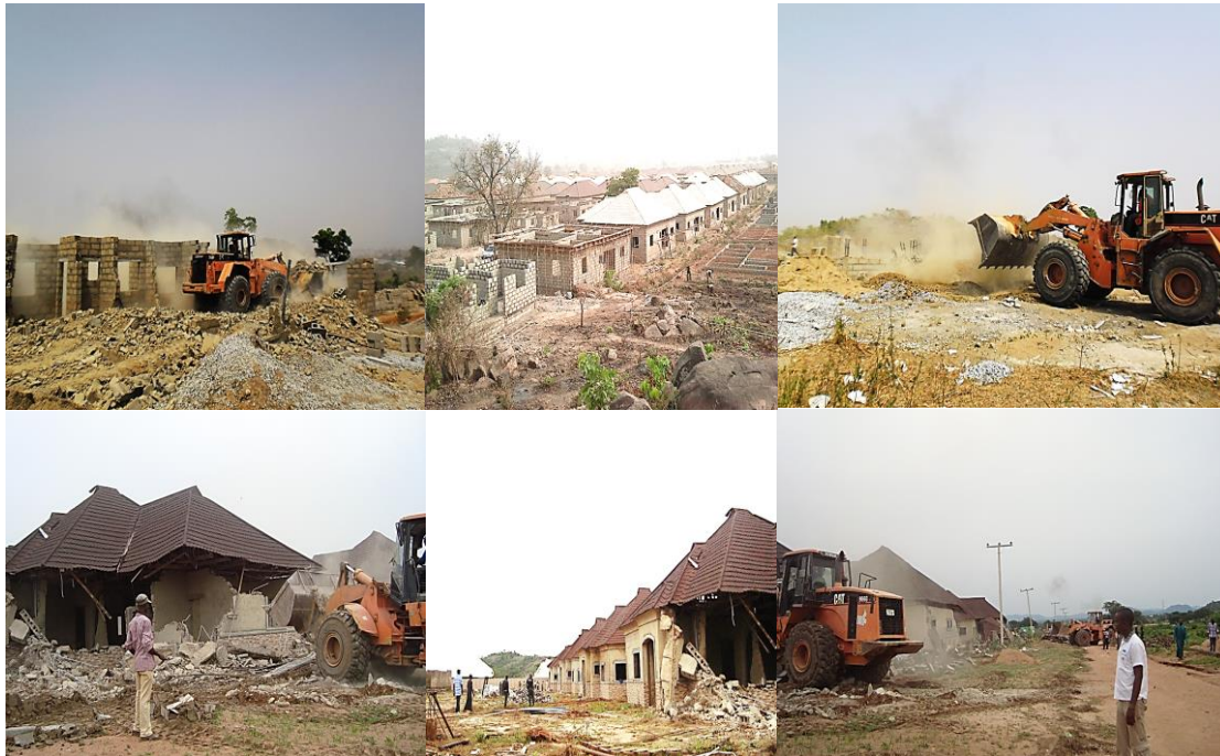
Figure 1: Bulldozers demolishing structures not in line with provisions of master plan; Author, 2013.
