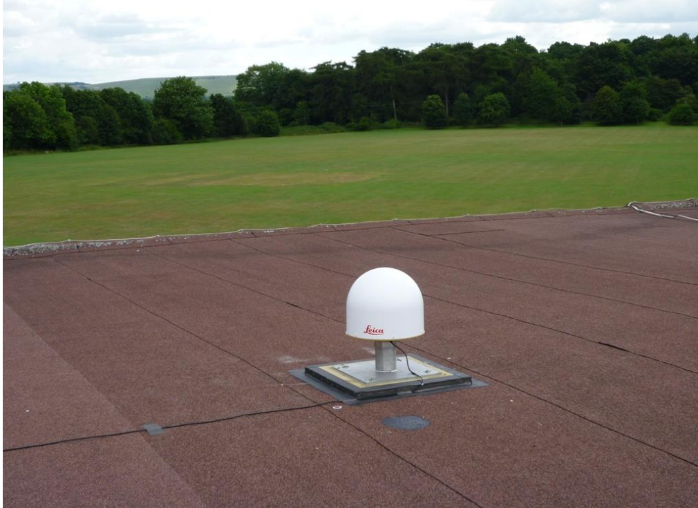
HUNG antenna installation which is approximately 5m above ground level.
