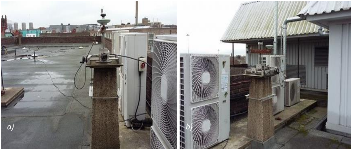
Figure 5.3: a) DRMS antenna environment looking North West. b) DRMS antenna environment looking North East.
