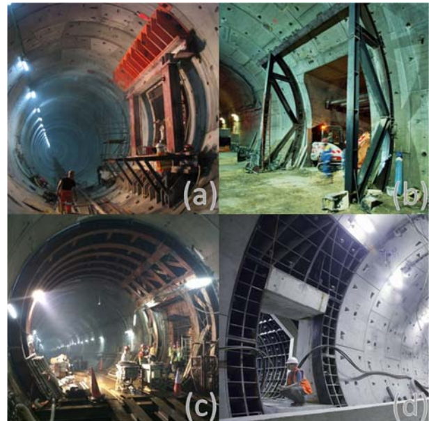
Figure 4. Temporary steel bracing structures for cross passages: a - steel lintel and sill beams; b - half-moon frame, c - full-moon frame, d - rectangular frame of steel segments (modified from Lee and Choi)
