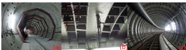
Figure 11. Protection measures for tunnels in close proximity - Temporary bracing (a) Supplementary grouting (b) Ductile segment (c) (from Chang et al.)
