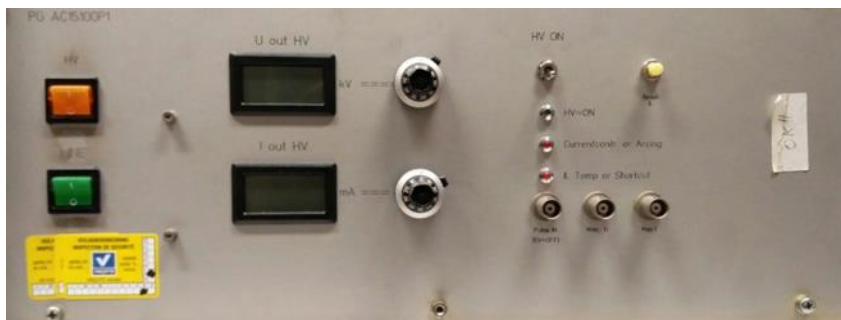
Figure 3.5. Photo of AC power source
