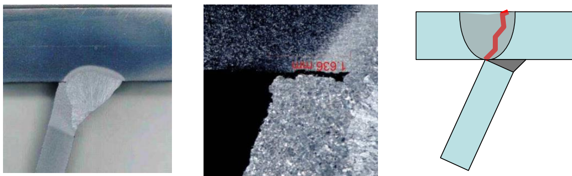
Fig. 4. (left) single side welding (centre) detail of stiffener (right) fatigue crack path
