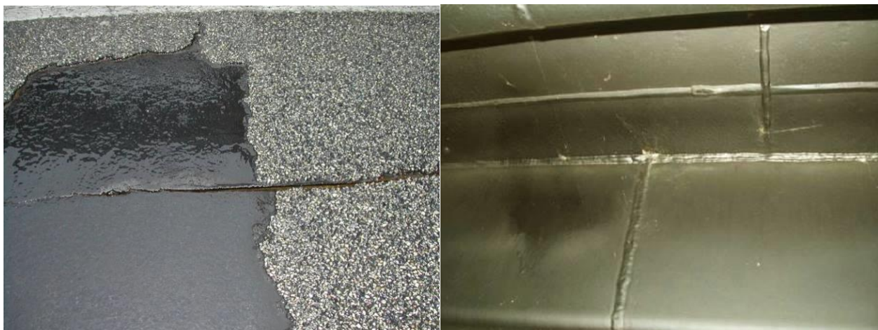
Fig. 3. Crack in deck plate (left) interference with stiffener butt weld (right)
