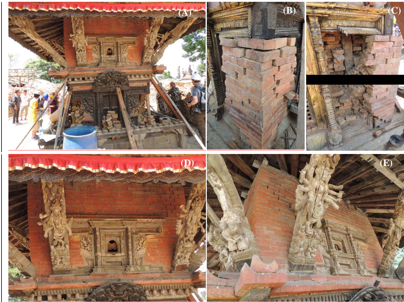
Fig. 8 - Kileshwar Mahadev temple: (A) Collapsed masonry at corners; (B)-(C) Dislodged outer leaf; (D) Shear cracks and dislodged masonry in north wall at first floor level and (E) Split in the timber strut of the west wall.
