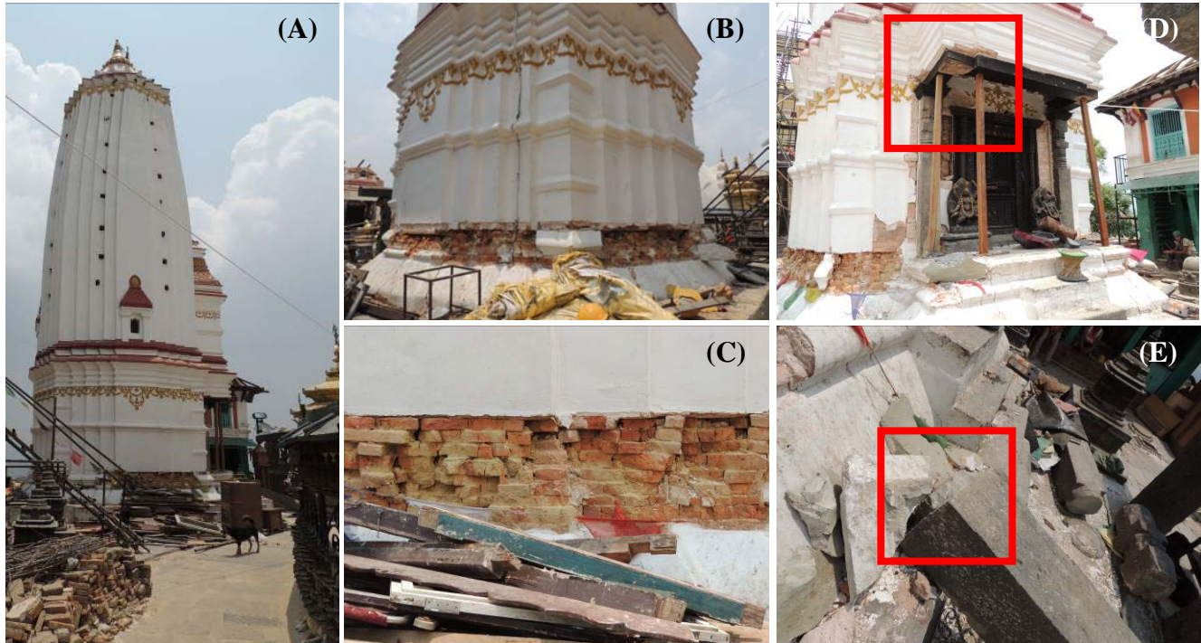
Fig. 3: (A) Pratappur Temple; (B) Damage to masonry plinth; (C) Crushing of brick masonry layers in mud mortar; (D) Collapsed portico of the temple; and (E) Lack of good connectivity at stone pillar base
