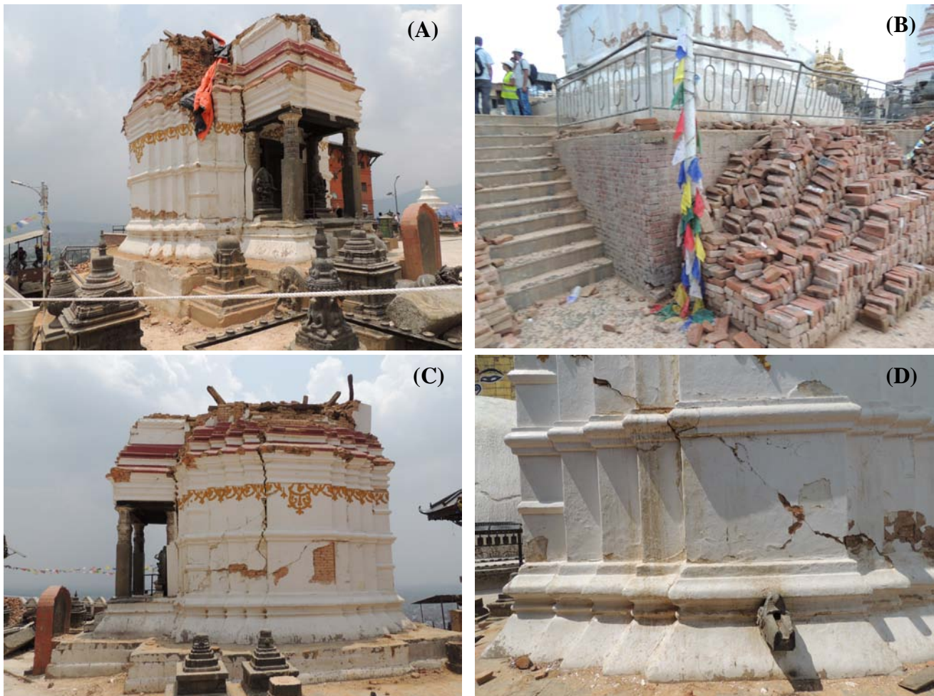
Fig. 4: (A) Anantpur Temple with collapsed shikhara; (B) Rear view of the structure showing repaired plinth; (C) Vertical cracks showing dilation of the structure; and (D) Shear cracks on the rear wall.
