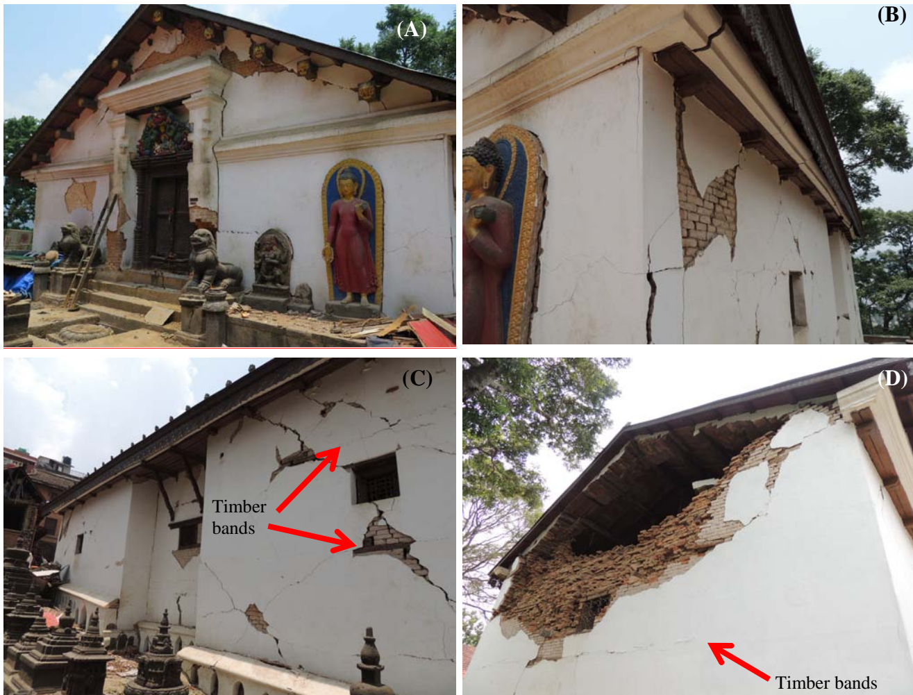
Fig. 10 - Shantipur temple: (A) Front facade (south); (B) Eastern facade showing out-of-plumb; (C) Eastern facade showing in-plane shear cracks and timber bands and (D) Rear facade with out-of-plane gable failure.
