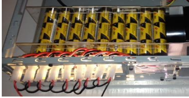
Figure 2: NiMH battery pack consisting of nine modules
