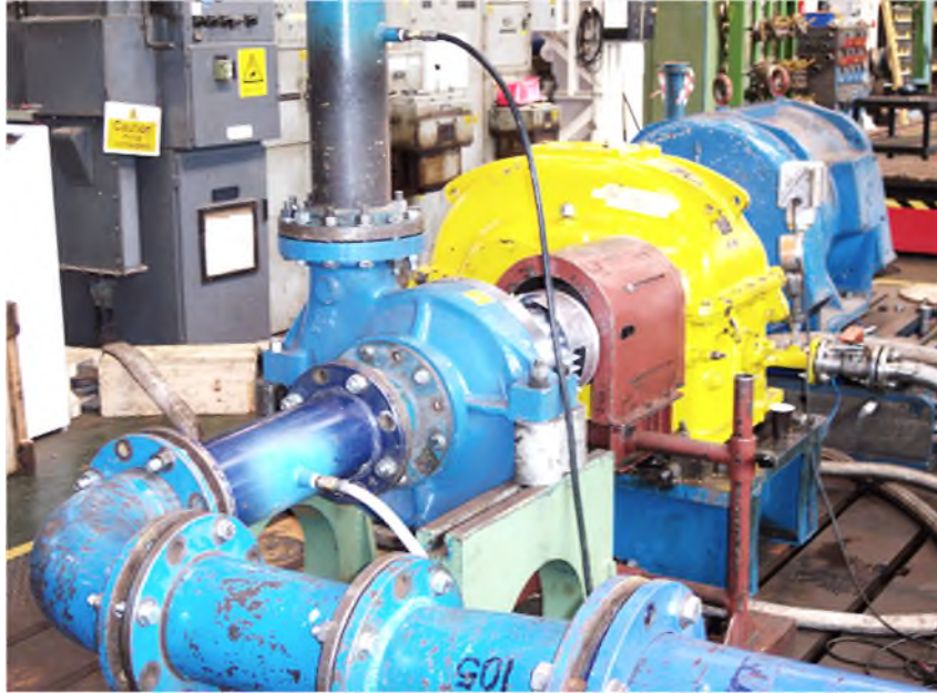
Figure 27 Photograph of the test pump set up on the test bed
