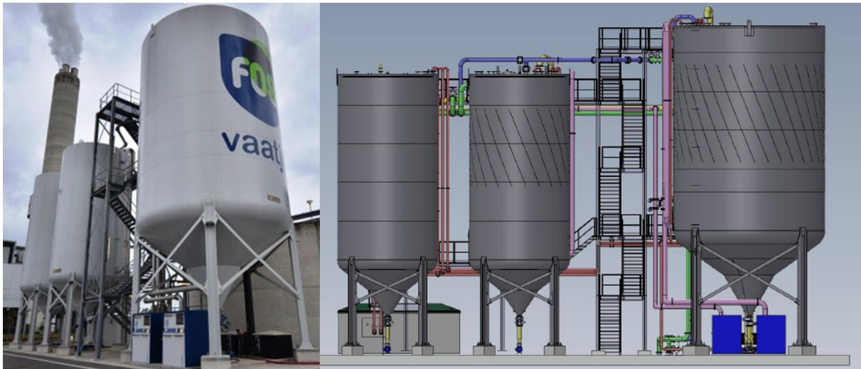
Figure S3: The Airprex ® reactor at WWTP Amsterdam west (Veltman, 2016)
