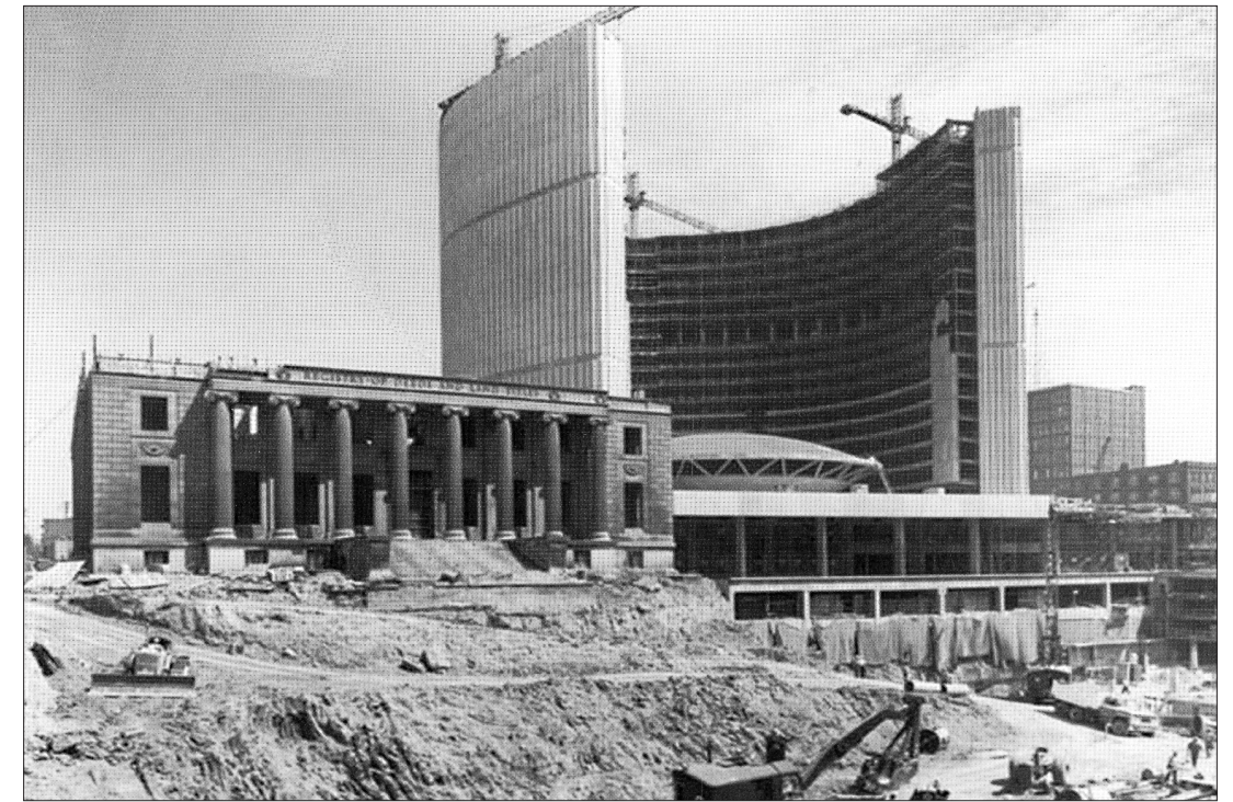
FIG 2 Postcard captioned, 'New City Hall under construction June 22nd, 1964', Canadian Architectural Archives
