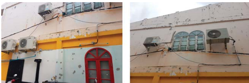
Figure 1. Air conditioning units arranged on low income housing units in Phuket, Thailand.
