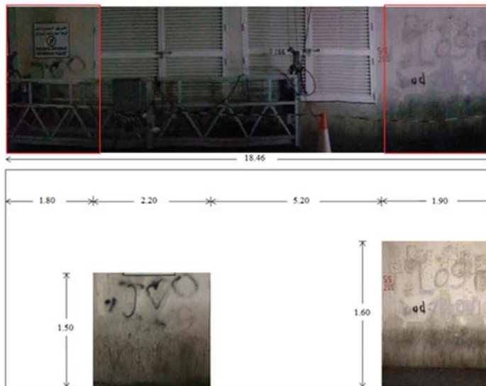
Figure 3. Image illustrating the width and height in meters of the vandalised wall in corridor A.
