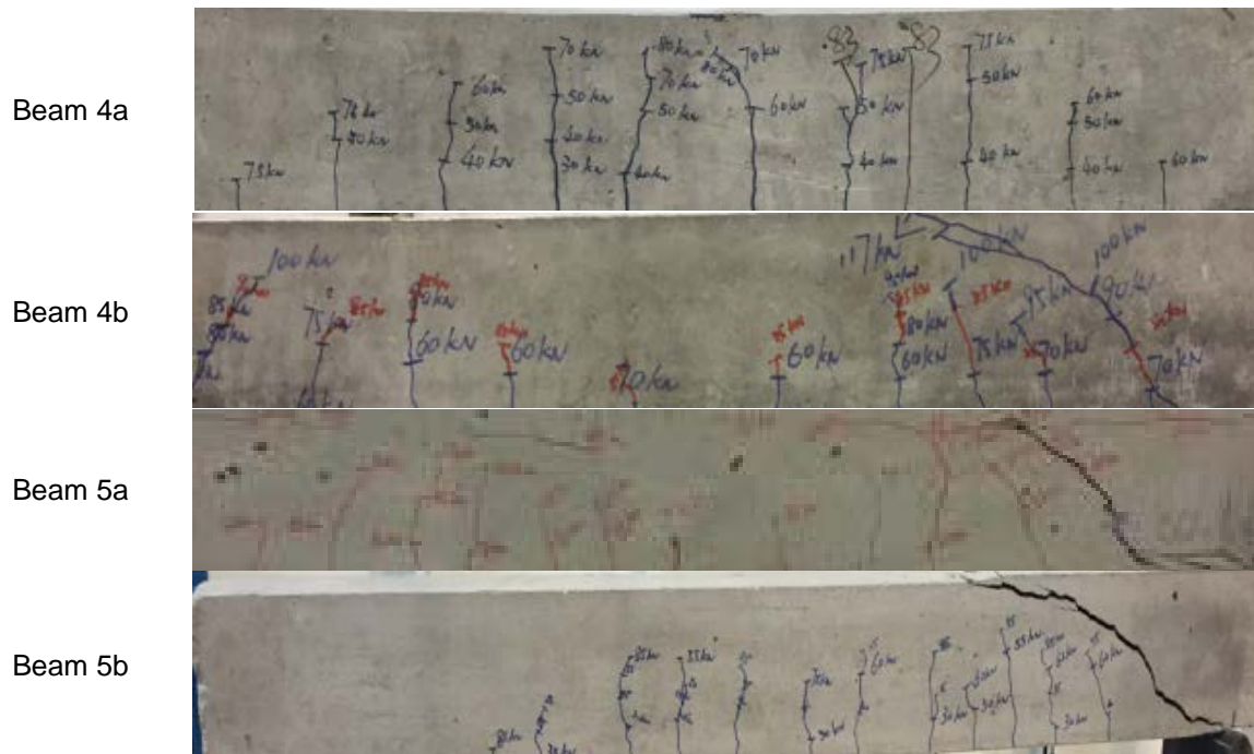
Fig.11. Crack patterns upon failure for four different beam types
