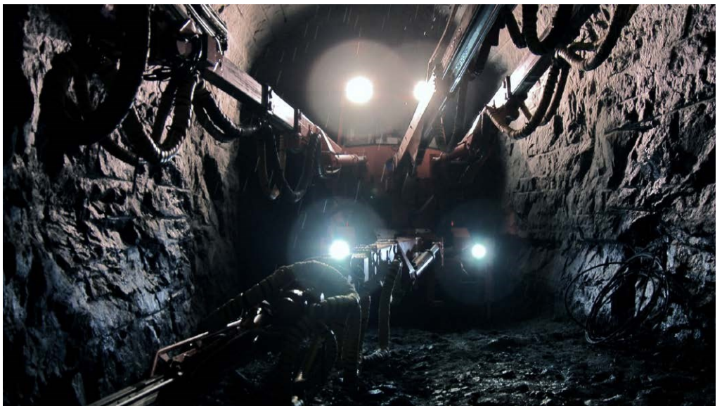
Figure 5. Work on the construction of the repository at ONKALO. Still from Into Eternity. Courtesy of Michael Madsen. Cinematography by Heikki Färm. Produced by Magic Hours Films. Used with kind permission.
