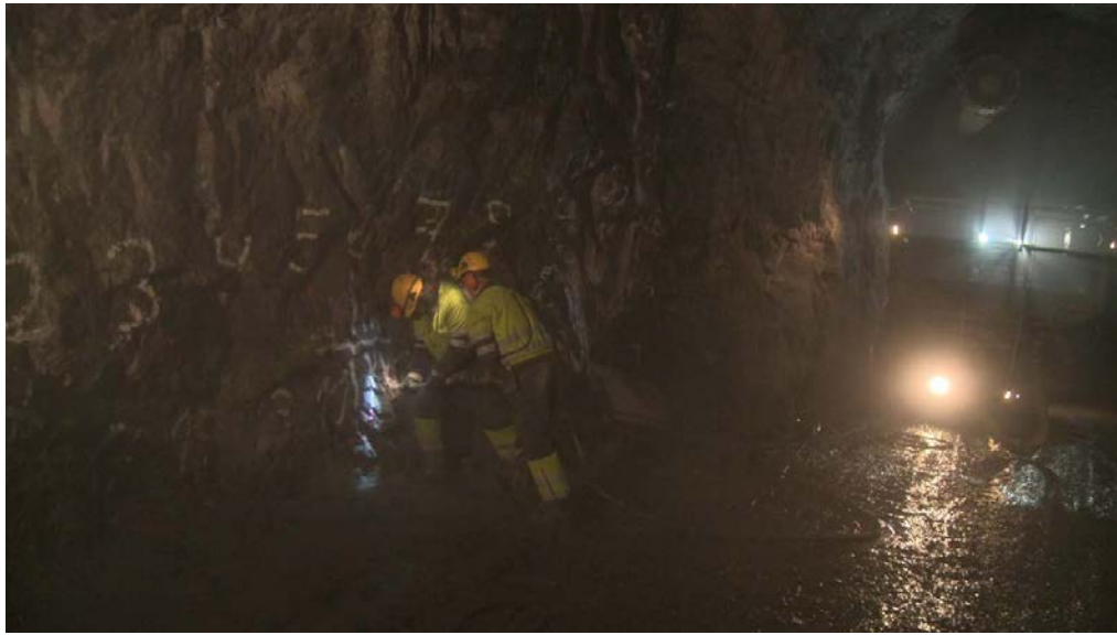
Figure 4. Work on the construction of the repository at ONKALO. Still from Into Eternity. Courtesy of Michael Madsen. Cinematography by Heikki Färm. Produced by Magic Hours Films. Used with kind permission.
