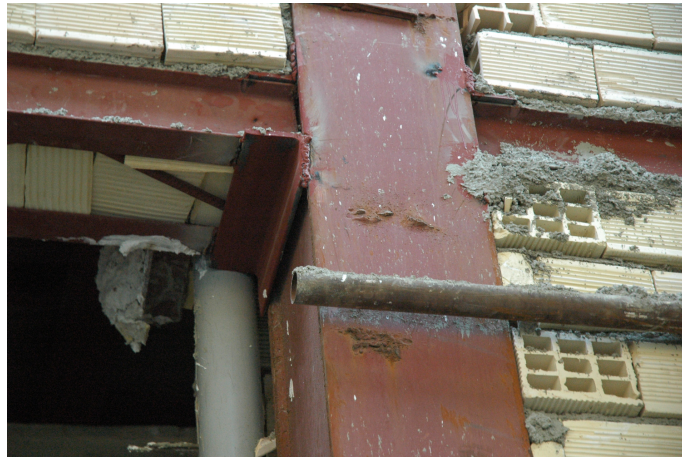
Figure 6: Human interference could increase the risk of defects, Source: the authors
