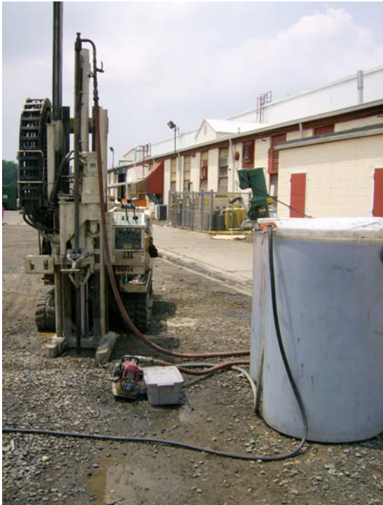
Figure 2 - Direct Injection of Iron NPs in the Field at the Trenton Facility, New Jersey (Photo courtesy of Geosyntec Consultants)
