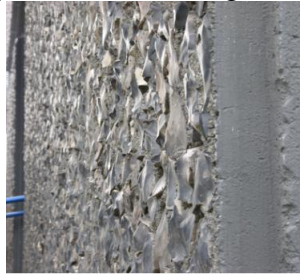
Fig.1b. Flint wall, Cockroft building, University of Brighton (UoB). Photo taken by Mr H. Hills, SET, UoB
