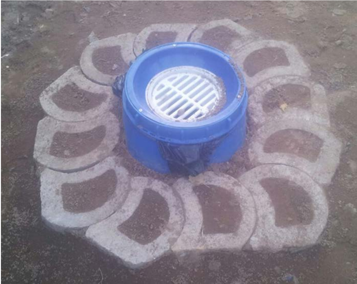
Figure 3: A ad hoc sewer implemented by the GoS team. Previous ad hoc sewers did not contain a removable sieve, making the system prone to clogging ( http://www.acturban.com/genius-of-space-berg-river/ , accessed 1/10/2016).
