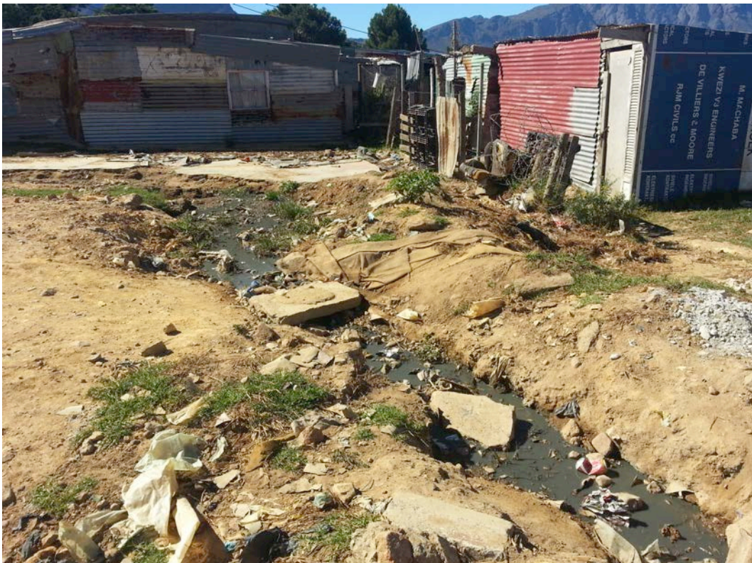
Figure 2: A typical scene in Langrug, where sewers get clogged with solid waste, resulting in stagnant contaminated water.
