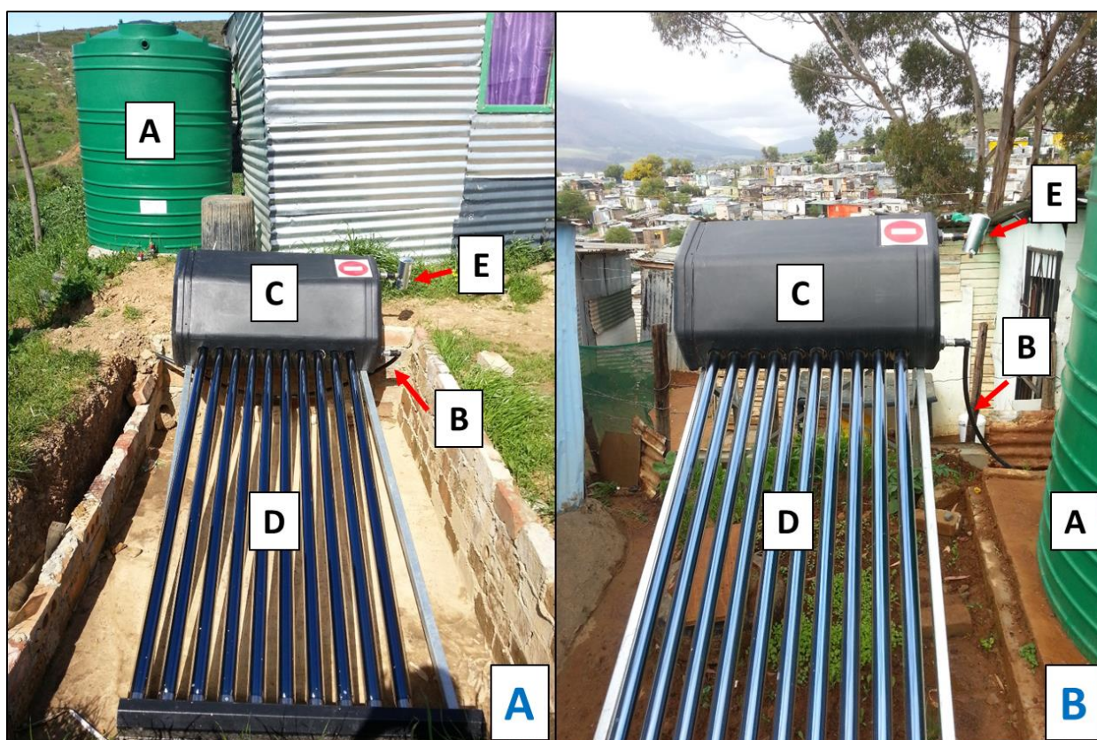
Fig. 2.1. (A) Small-scale SOPAS system installed at Site 1. (B) Small-scale SOPAS system installed at Site 2. The labelled system components are: (A) rainwater harvesting tank, (B) pipe connecting rainwater tank to SOPAS system, (C) storage tank of SOPAS system, (D) high borosilicate glass tubes, (E) outlet tap.
