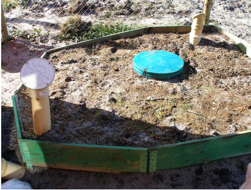
Photo 4.16: External view of biodigesting unit (Site B)
