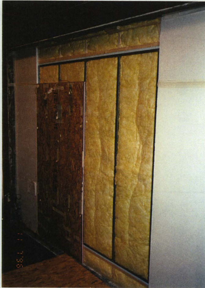
Figure 4-8, FSEC metal-wood wall installed in guarded hot box test facility at ORNL for thermal testing.
