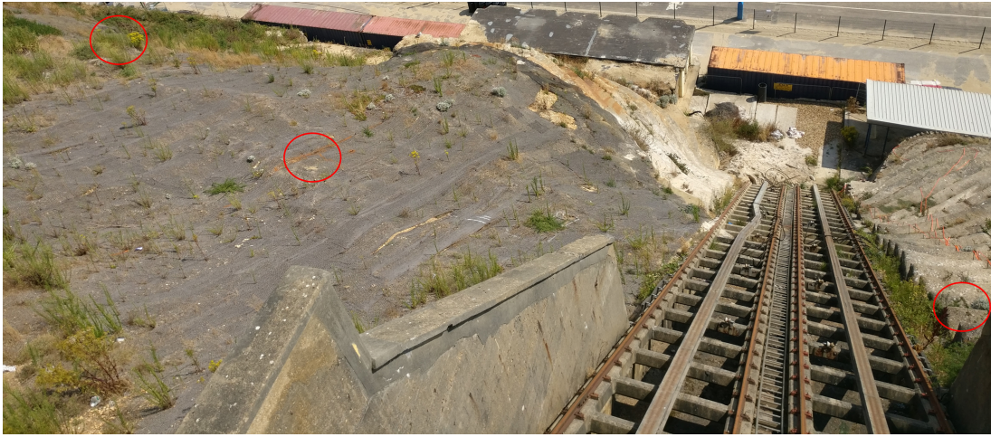
Fig. 5. The landslide area where the IoT-enabled monitoring system has been deployed. The landslide has taken place in the area on the left of the rails. At the top of the picture, the damaged public access buildings are visible, as well as the damage inflicted on the rail of the rail-wagon (used to facilitate public access to the beach). The red circles denote the positions of the installed sensing devices.
