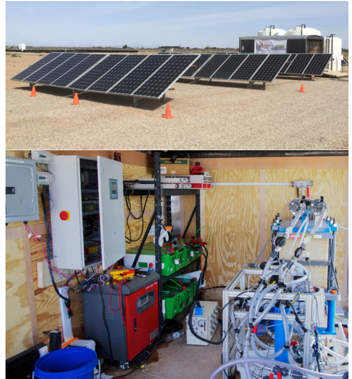
Figure 5: The prototype system at BGNDRF showing full system with panels, trailer, and water tanks (top). All electronic control, battery storage, and hydraulic subsystems were installed inside the trailer (bottom).
