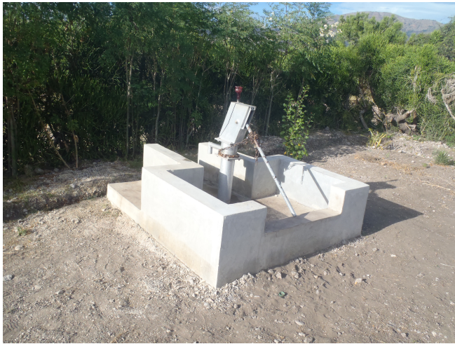
FIGURE 1. The Bercy well as installed by CHI Haiti.
