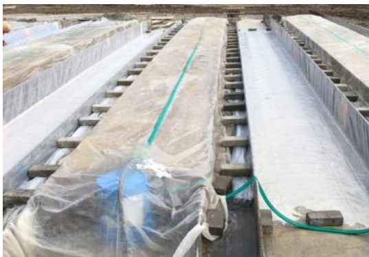
(a) Simple steel forms to cast planks (photo taken at the Midwest Underground Casting Facility in Nebraska)
