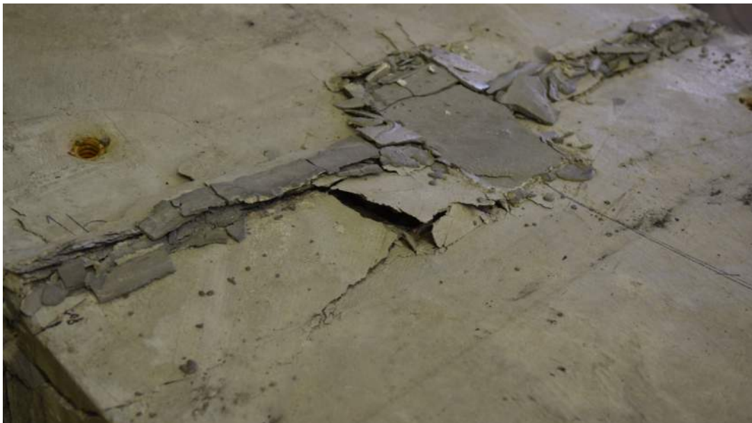
Figure 3.16: Specimen F-F-1 Joint Close-up Photo after Failure
