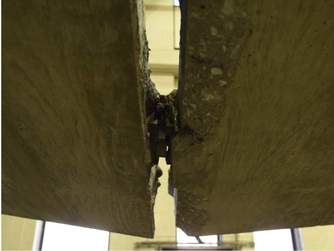
Figure 3.17: Mechanical Joint Connecting the adjoining Slabs after Failure
