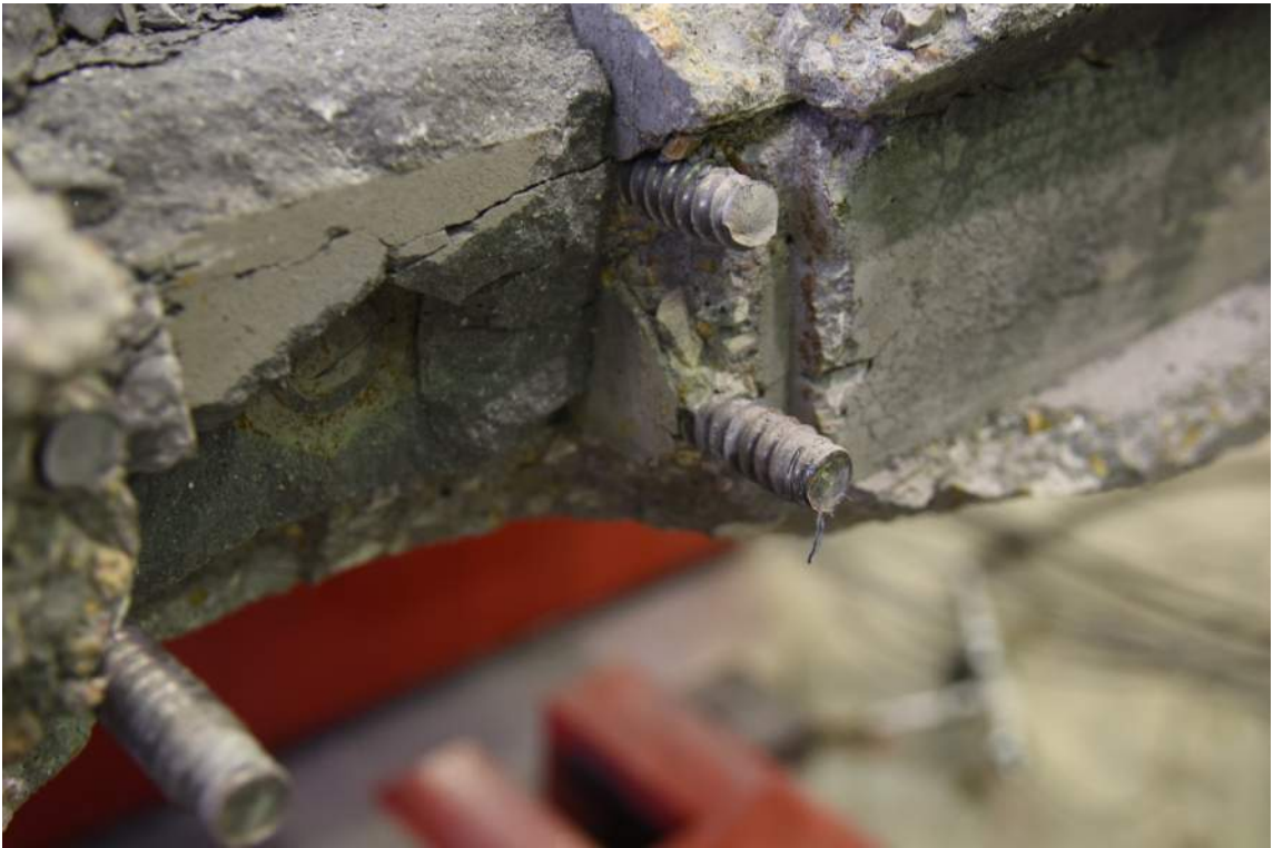
Figure 3.24: Mechanical Joint Shear Failure (Specimen C-C-1)
