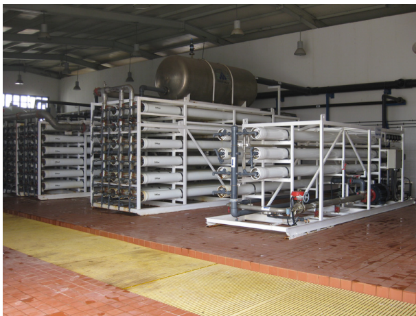
Figure 8. Dahab RO Membrane Unit
