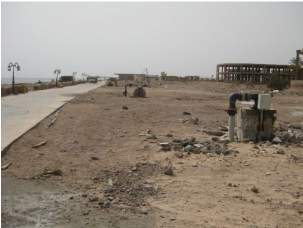
Figure 7. Well field at Dahab desalination plant
