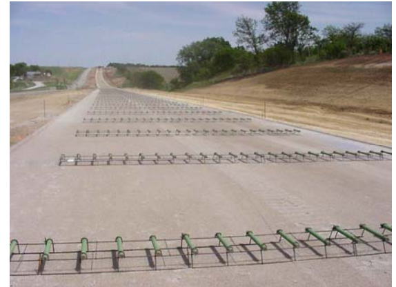
Dowel bars placed on chairs ready for paving. (Photo compliments of Lieska Halsey)
