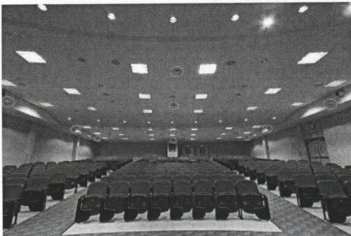
Figure 1. Overhead coverage deployment in lecture hall
