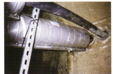
Figure 6. Results after less than three days of repair work. The cable pairs are spliced and sealed in an airtight case. A brace is installed to prevent the weight of the cable from breaking the splices. A maintenance tag is applied to the splice box to indicate the last time the splice box was checked. Manholes should be periodically checked to prevent deterioration of the splices.
