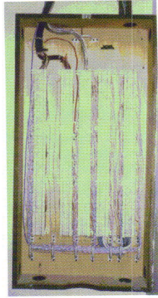
Figure 4. Results after less than one day of repair work. Jumper wires are properly secured. It is very easy to determine port availability.
