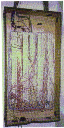
Figure 3. Before picture of a typical intermediate distribution frame (wiring closet). Jumper wires are run point-to-point and not through any D-rings.
